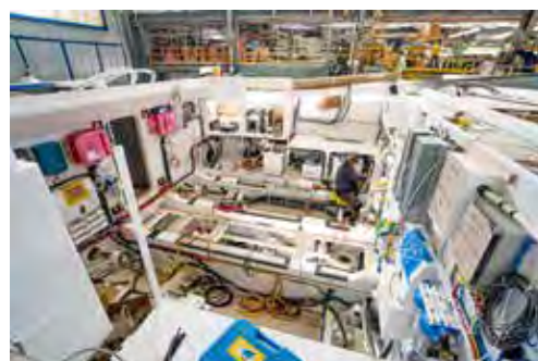
ROUGH ELECTRICAL The 92 Convertible Engine room.
